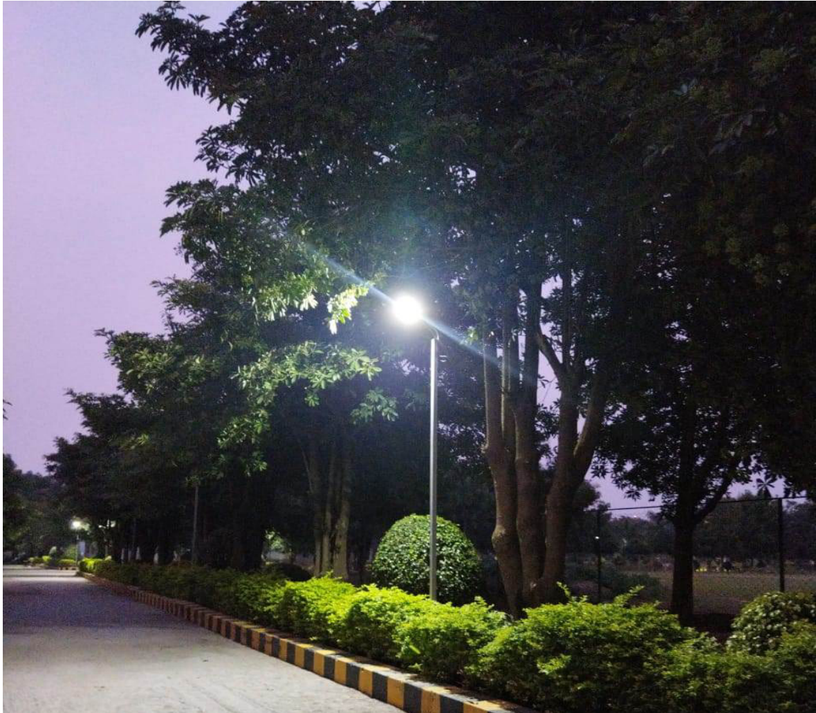
Sensor-Based solar power street lights in Campus Premises.
